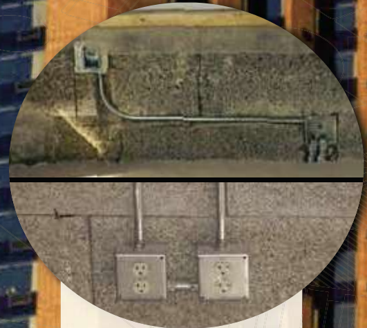
Accommodates electrical wires and services, either on or within the Nexcem surface
